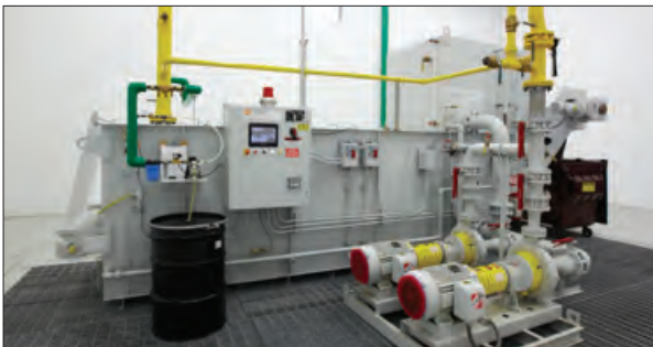
Rolled media vacuum filter installed in a bearing grinding operation, provides clean coolant plant wide.
